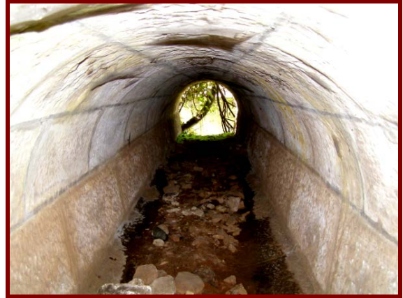
A well preserved culvert hidden beneath the old railway line below Pulpit Hill discovered on the walking tour, which probably dates to 1866.
