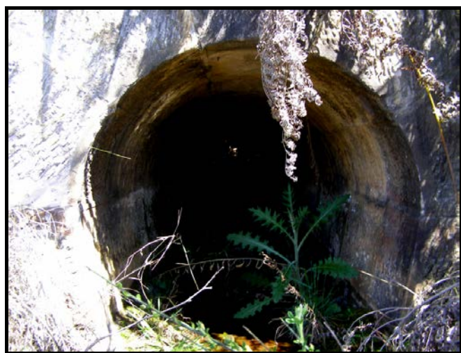
A second railway culvert found below the original single track railway constructed circa 1865, inside the proposed Pulpit Hill Heritage Precinct. Photograph taken 30-Sep-07.
